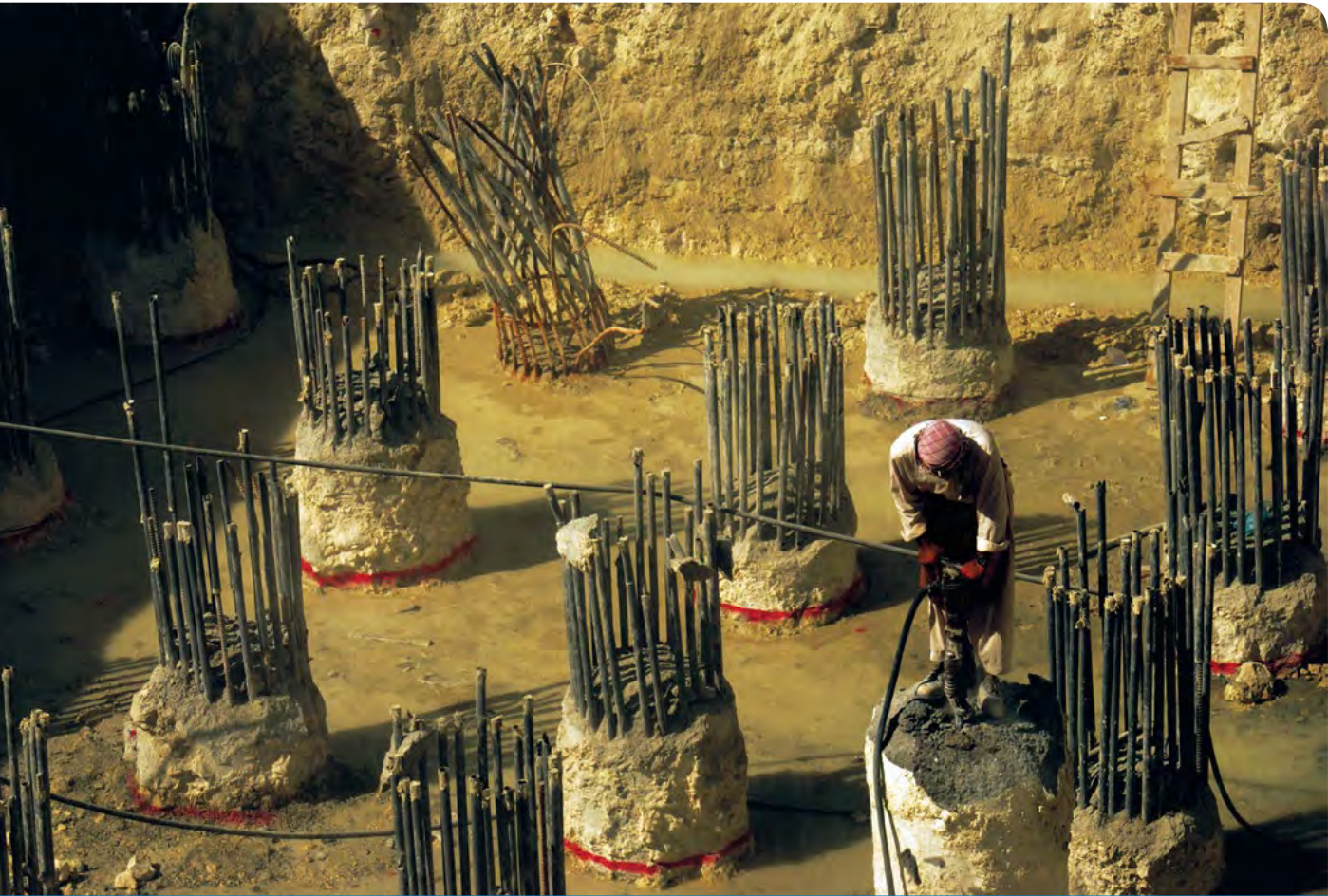
Construction work, Doha, Qatar. Photo by Dan A'Vard, reproduced under a CC BY-NC_SA 2.0 license.
